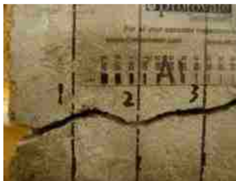
Figure 2.7 Typical corrosion-induced cracks on the concrete surface with a crack meter.
